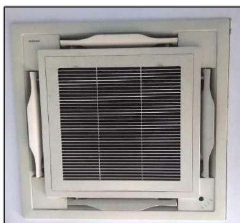
Fig. 6.3.6 Air Conditioners in LAB 3 (C514)
